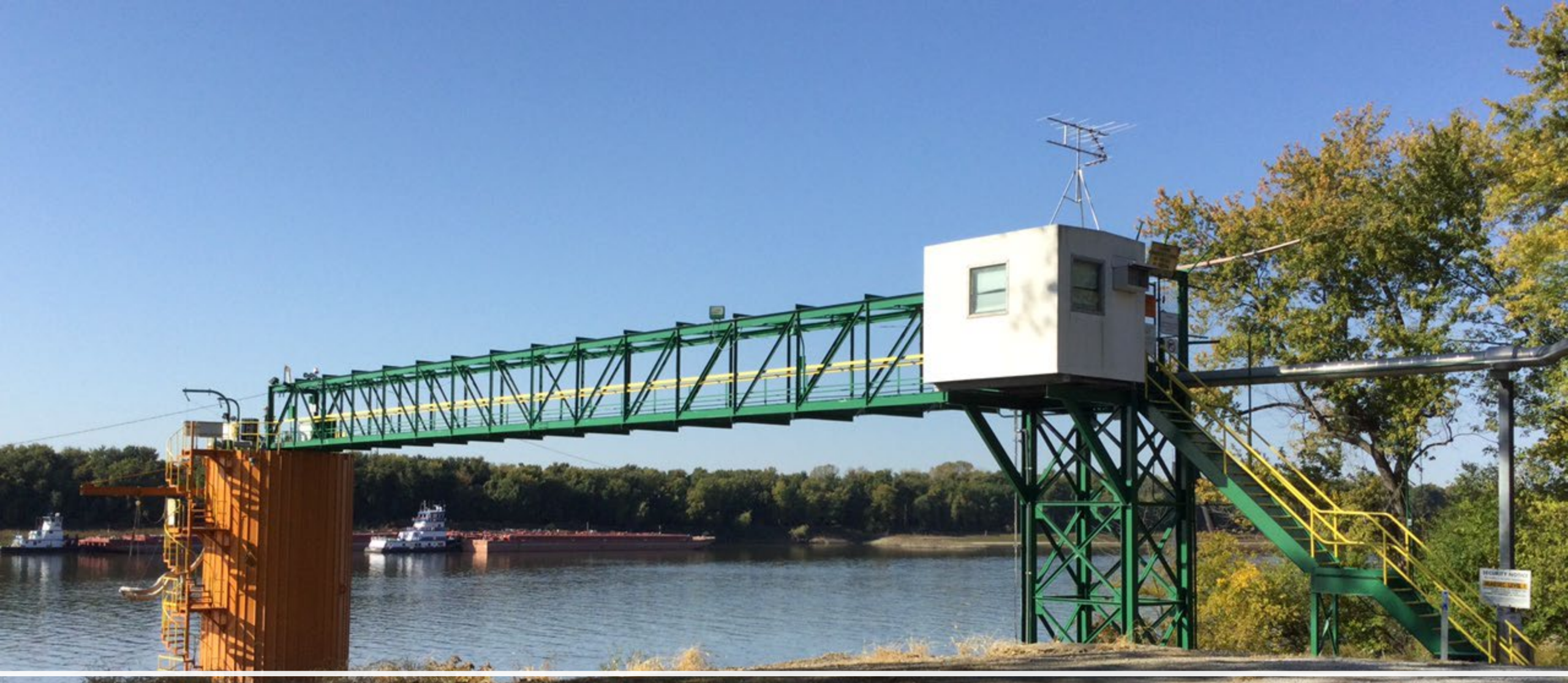
Anhydrous Ammonia Pipeline (at LDB)
